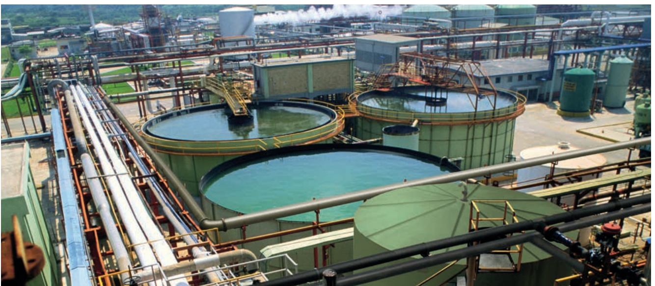
Rubber-lined sedimentation tank
