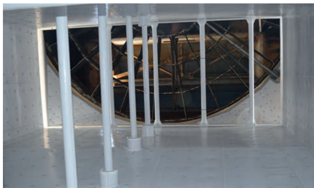
PFA lining in a raw gas duct
