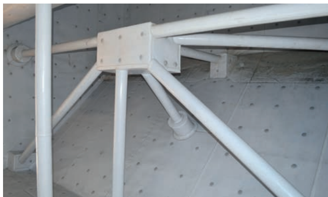
PFA lining in a raw gas duct
