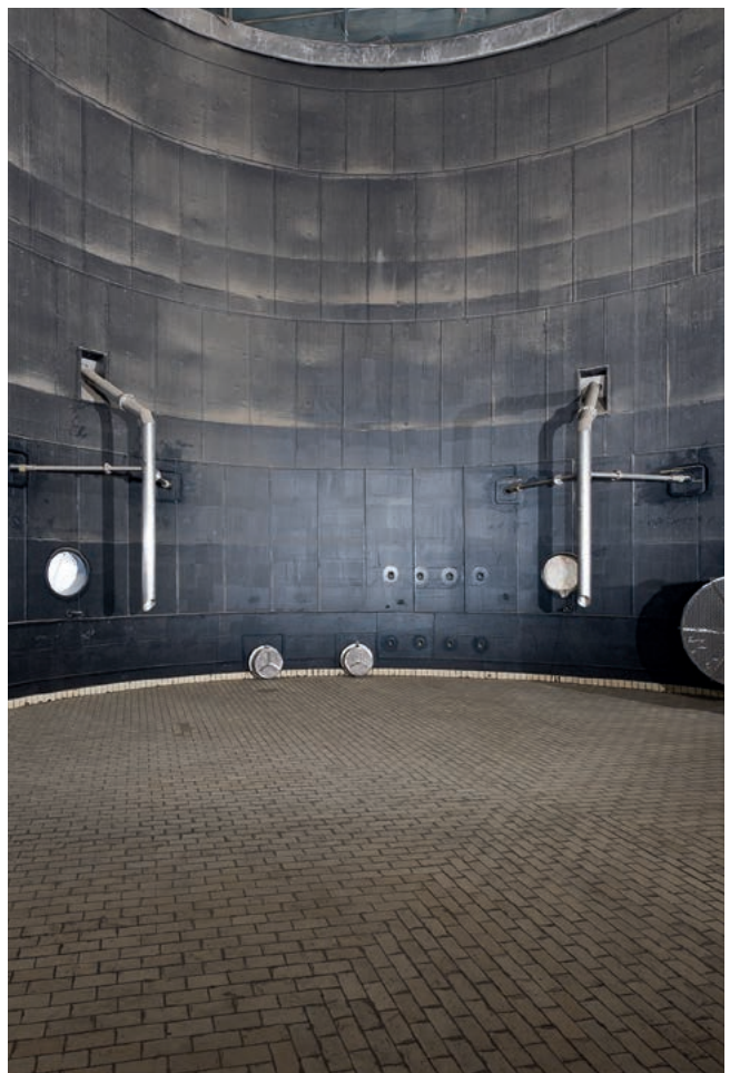
Rubber-lined flue gas scrubber
